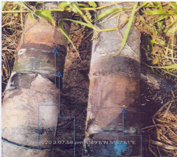
THREE HACKSAW CUTS ON THE FLOWLINE
